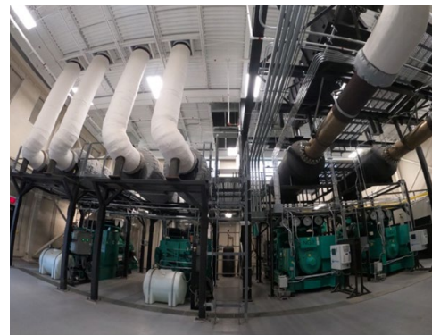
MCAS Miramar's Microgrid Mechanical Room
