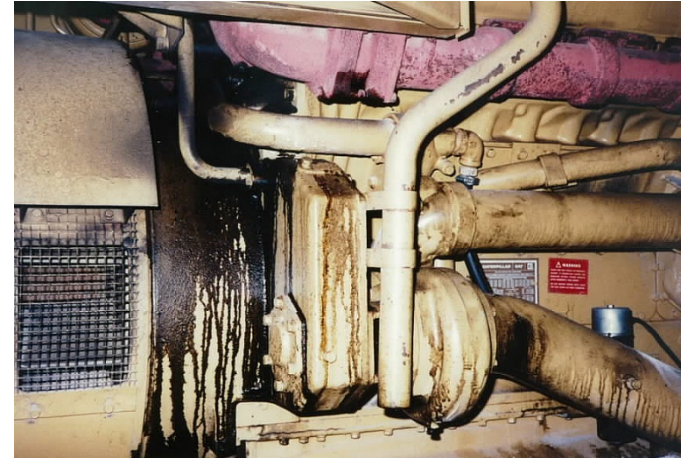
Wet stacking from unburned fuel
