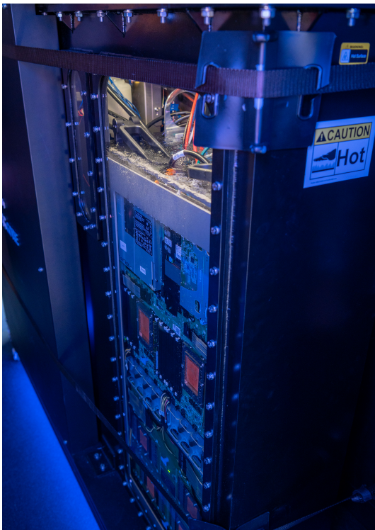
J-01: TMGCore's portable data center delivered computing capabilities at both Camp Roberts and the SLAMR site
