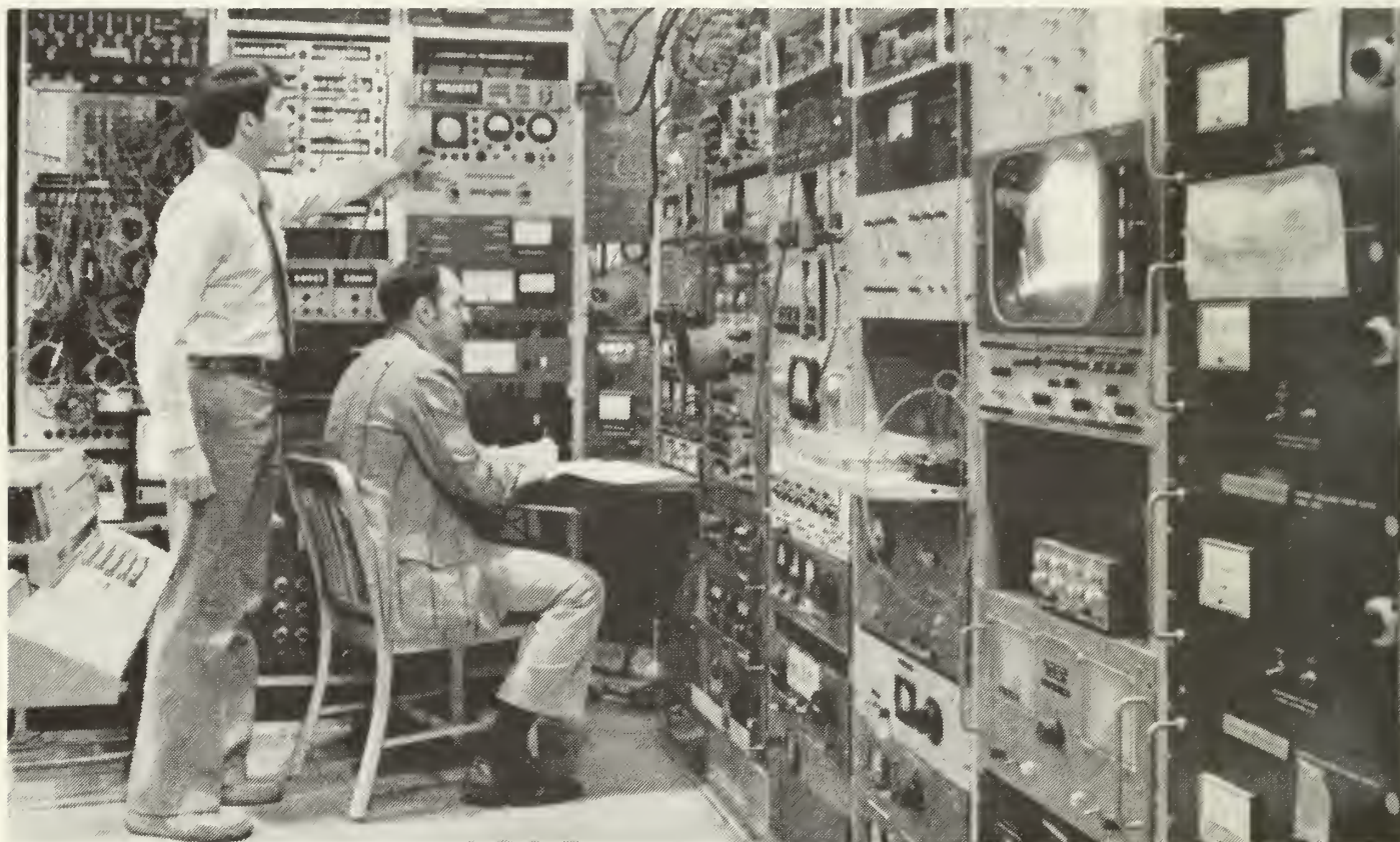
Control room of the Linear Accelerator
