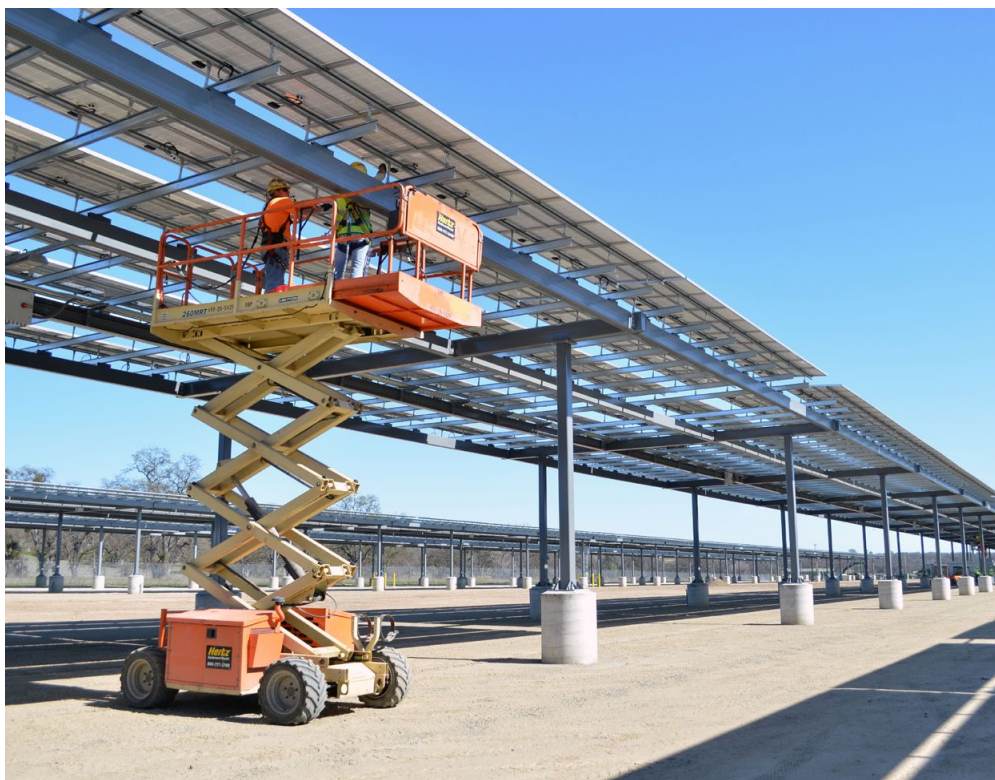
Solar microgrid project at Fort Hunter Liggett, California. (U.S. Army photo by John Prettyman)
